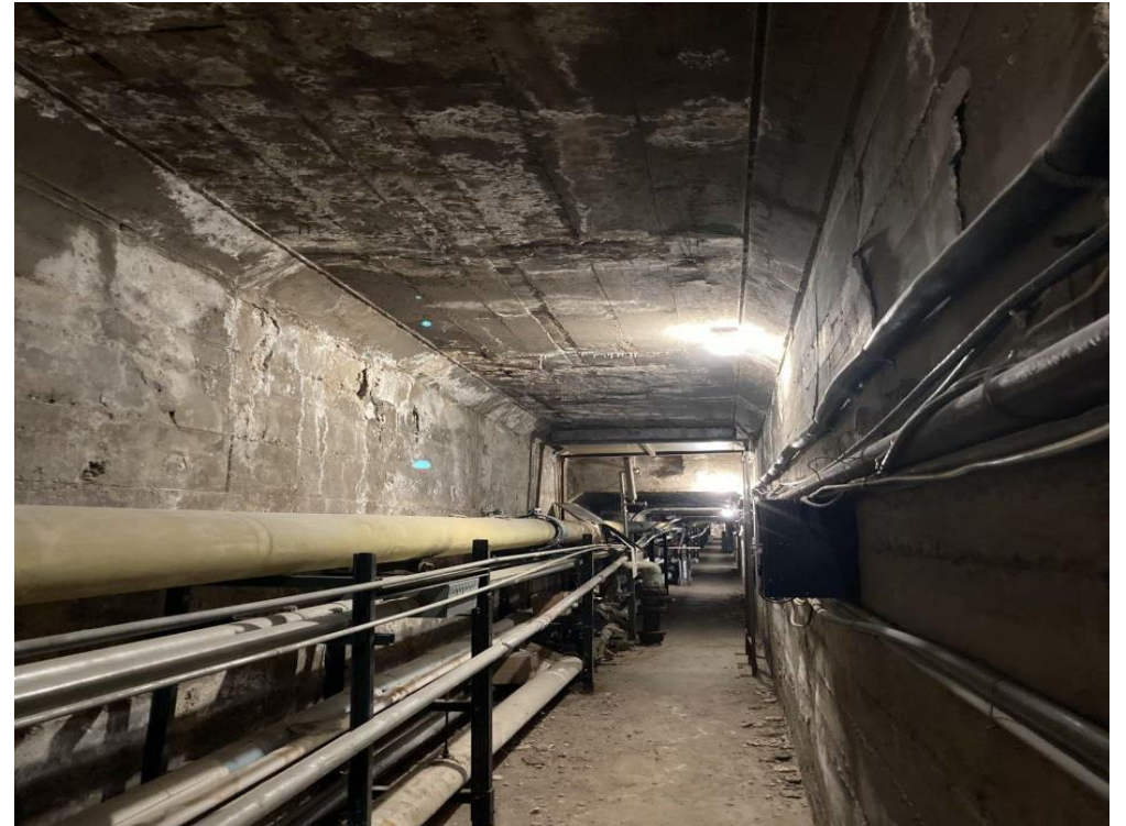
EXISTING TUNNEL - WITH VARIOUS INFRASTRUCTURE PROBLEMS
