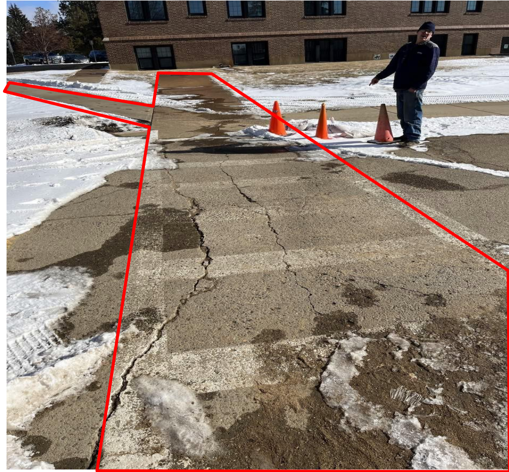
FOREGROUND SHOWS TOP OF EXISTING TUNNEL AS A CROSSWALK ON A PRINCIPAL DSU STREET. CONES AND SANDBAGS INDICATE AREAS OF SURFACE WATER SEEPING INTO TUNNEL. THIS STREET IS NOW CLOSED IN THIS AREA.
