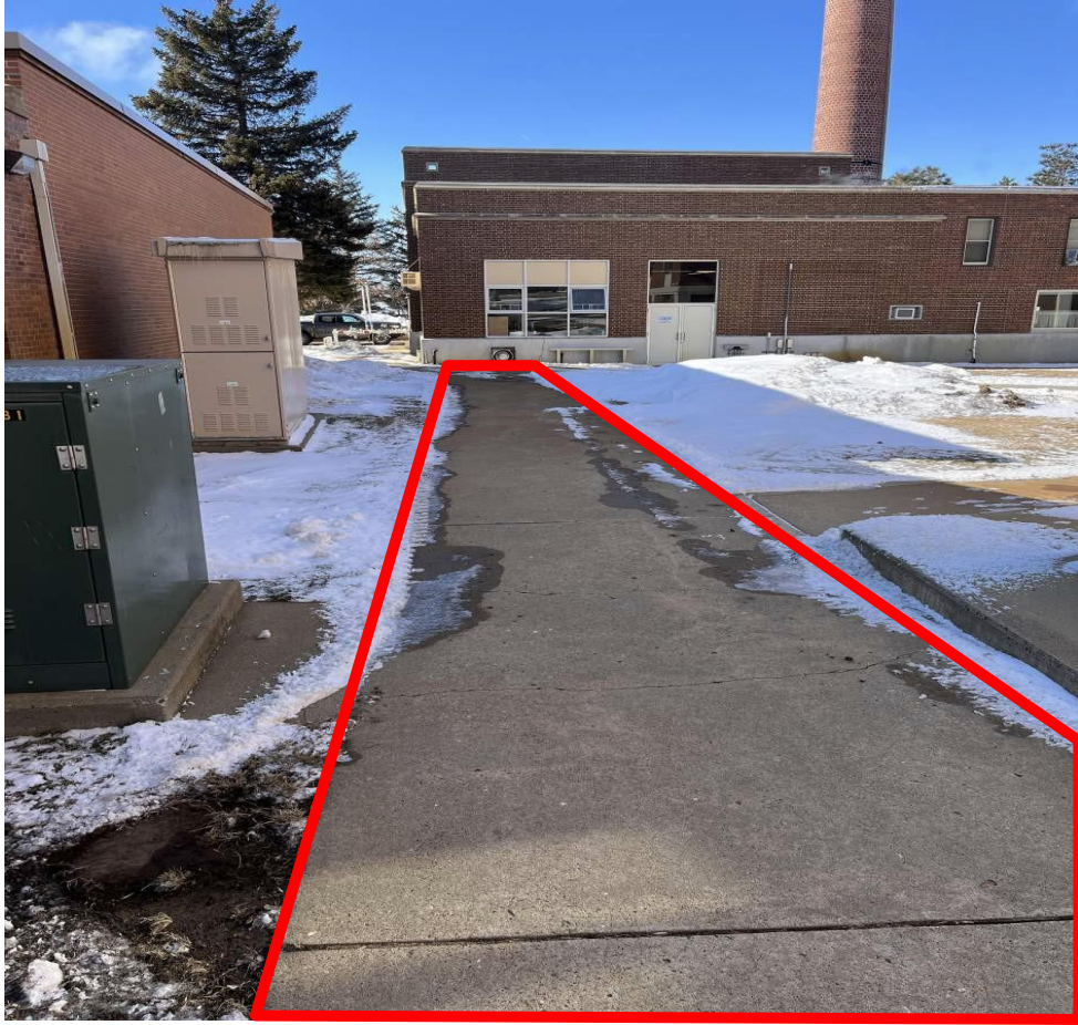
THE TOP OF THIS EXISTING TUNNEL IS A SIDEWALK THAT IS CLOSE TO MAJOR ELECTRICAL UTILITES
