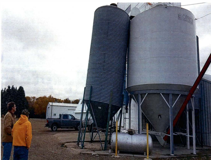
Old Holding Bin—Result of Failed Concrete
