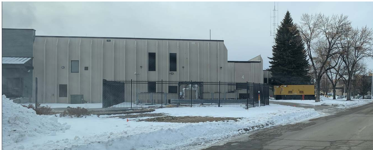
PHOTO SHOWING BOTH BACKUP GENERATORS AND HVAC EQUIPMENT (BEHIND FENCE). WHILE THE FENCE IS OF SUFFICIENT STRENGTH TO DETER VANDALS OR THIEVES FROM TAMPERING WITH THE EQUIPMENT, IT IS NOT STRONG ENOUGH TO PREVENT A VEHICLE FROM CRASHING THROUGH AND DAMAGING THE COOLING EQUIPMENT.
